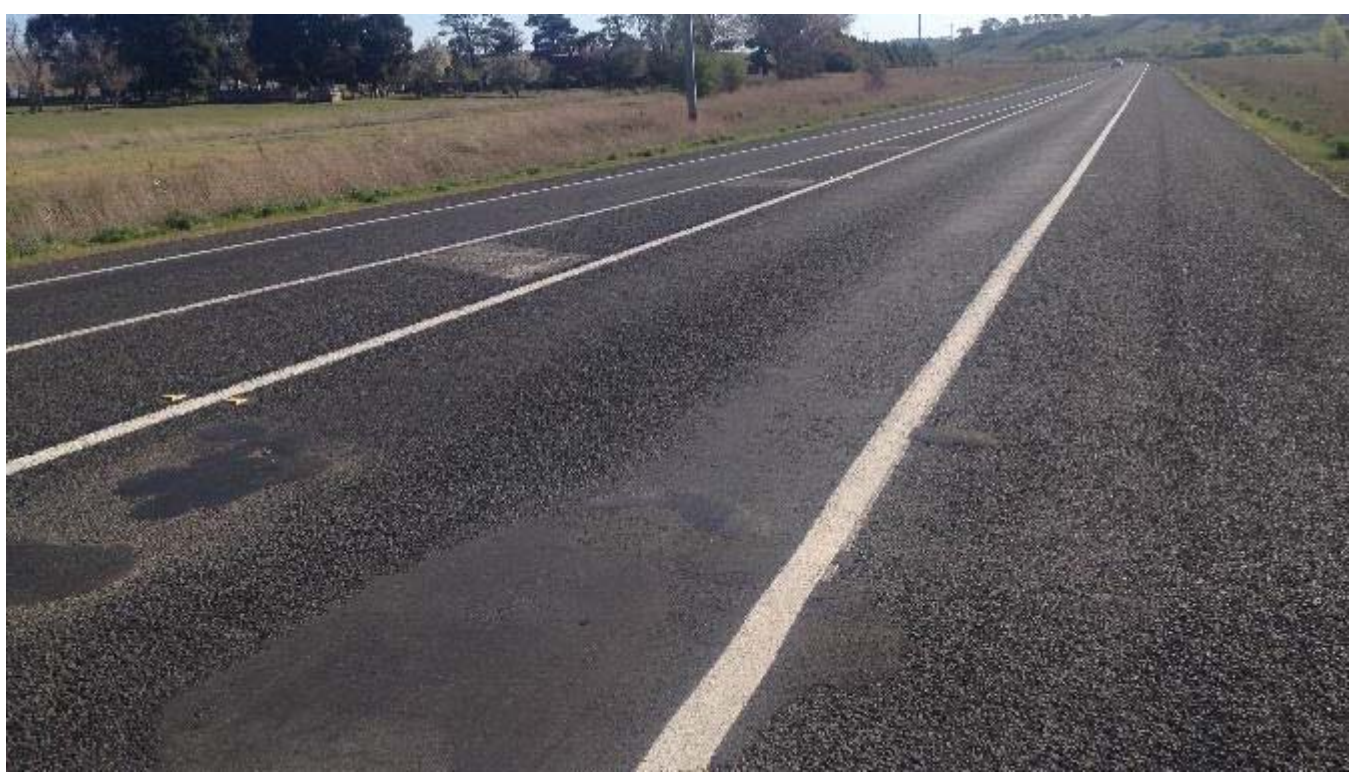
Plate 25: Stripping of aggregate, loss of texture and deformation – evidence of repaired potholes
