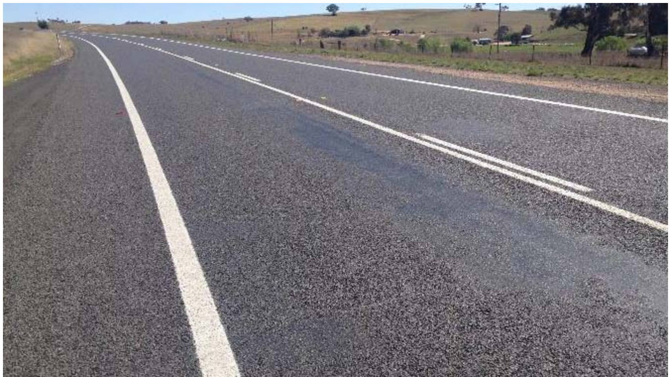
Plate 18: Stripping of aggregate and loss of texture – evidence of recent repair.
