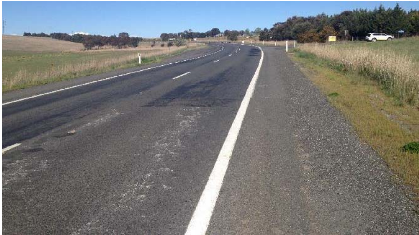
Plate 23: Block Cracking, stripping of aggregate, loss of texture and deformation
