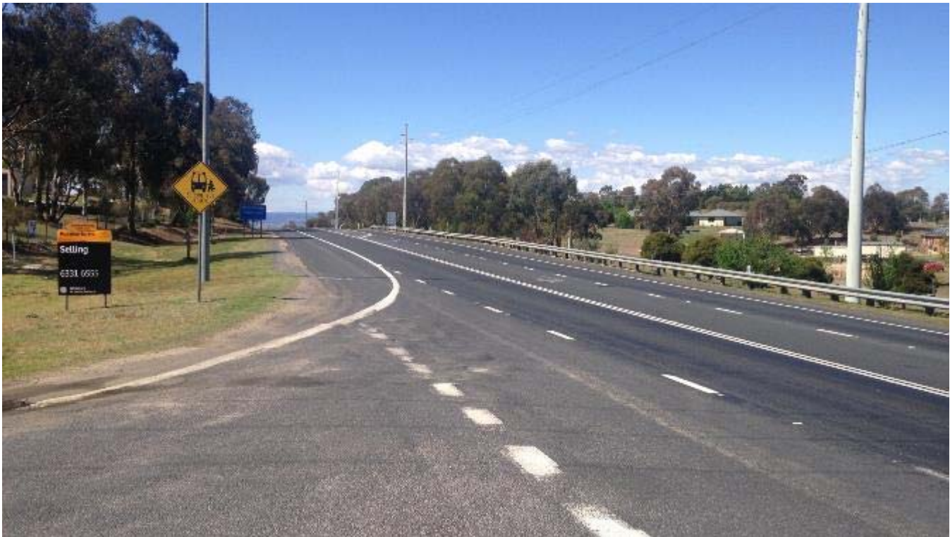
Plate 16: Minor stripping of aggregate, loss of texture and minor deformation.
