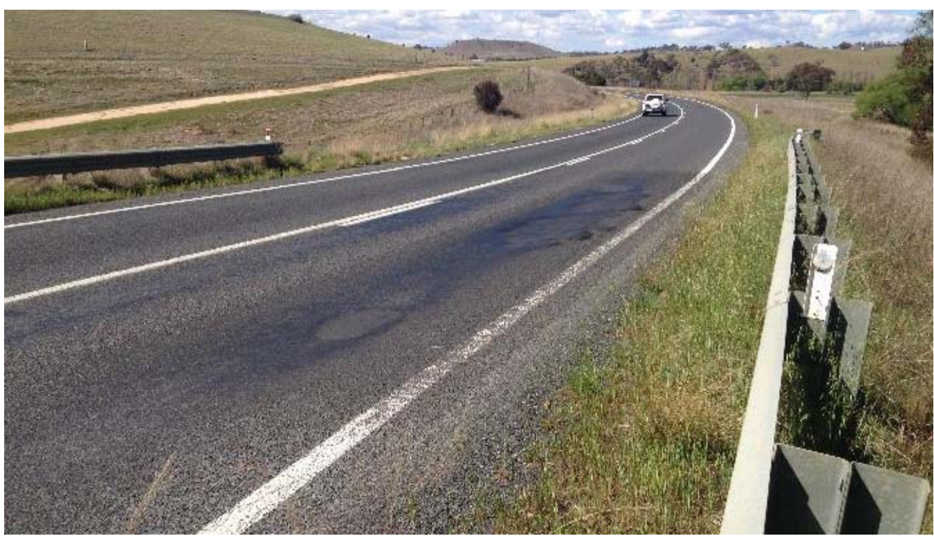
Plate 19: Block cracking, stripping of aggregate, loss of texture and significant deformation
