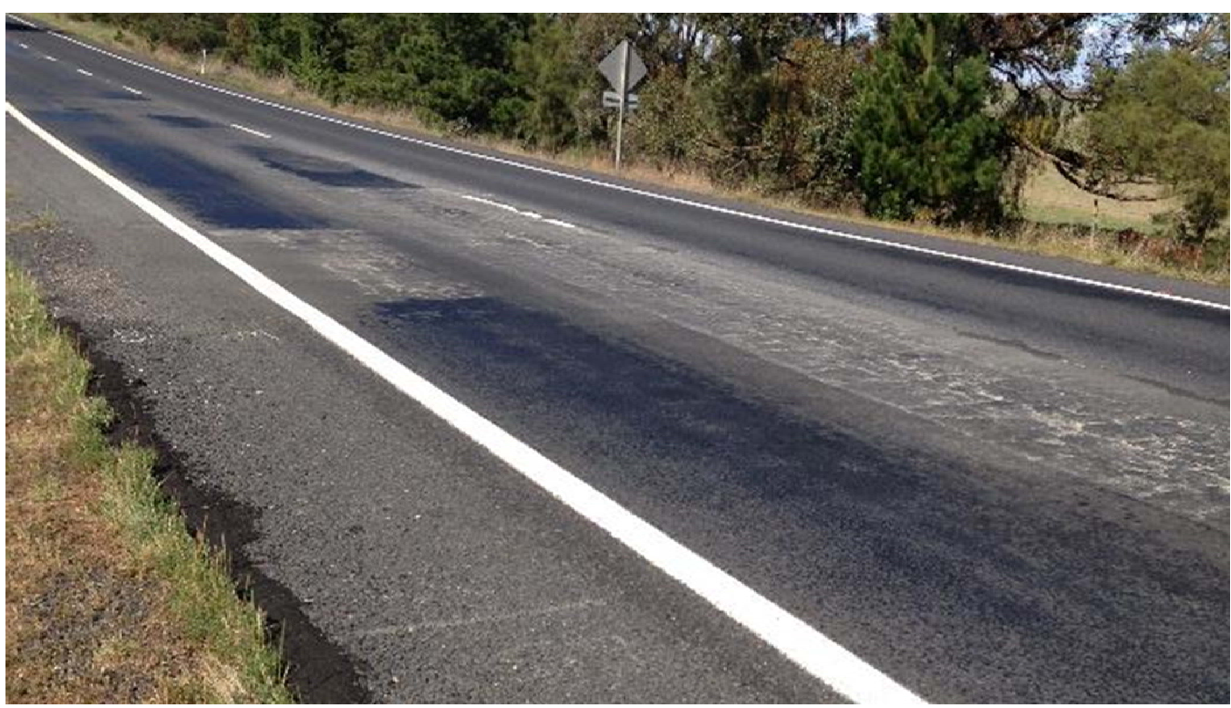
Plate 21: Block cracking, stripping of aggregate, loss of texture and some deformation – evidence of repairs
