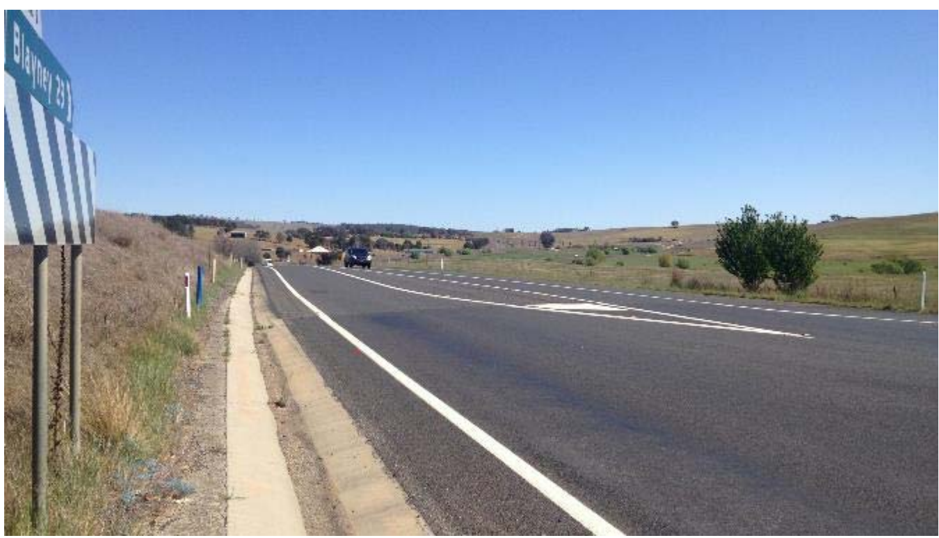
Plate 17: Minor stripping of aggregate and loss of texture – evidence of recent repair.
