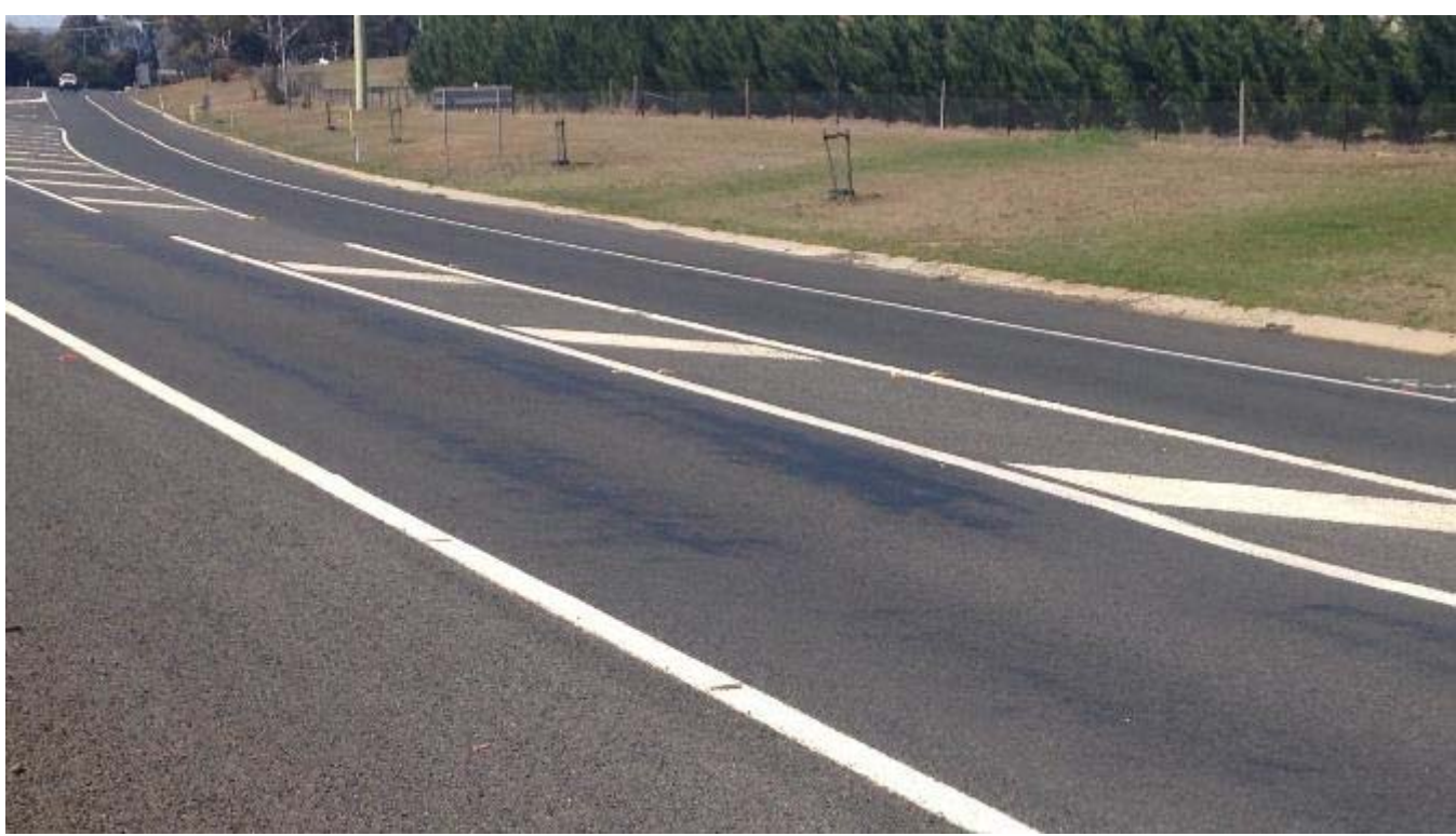
Plate 15: Minor stripping of aggregate, loss of texture and minor deformation.
