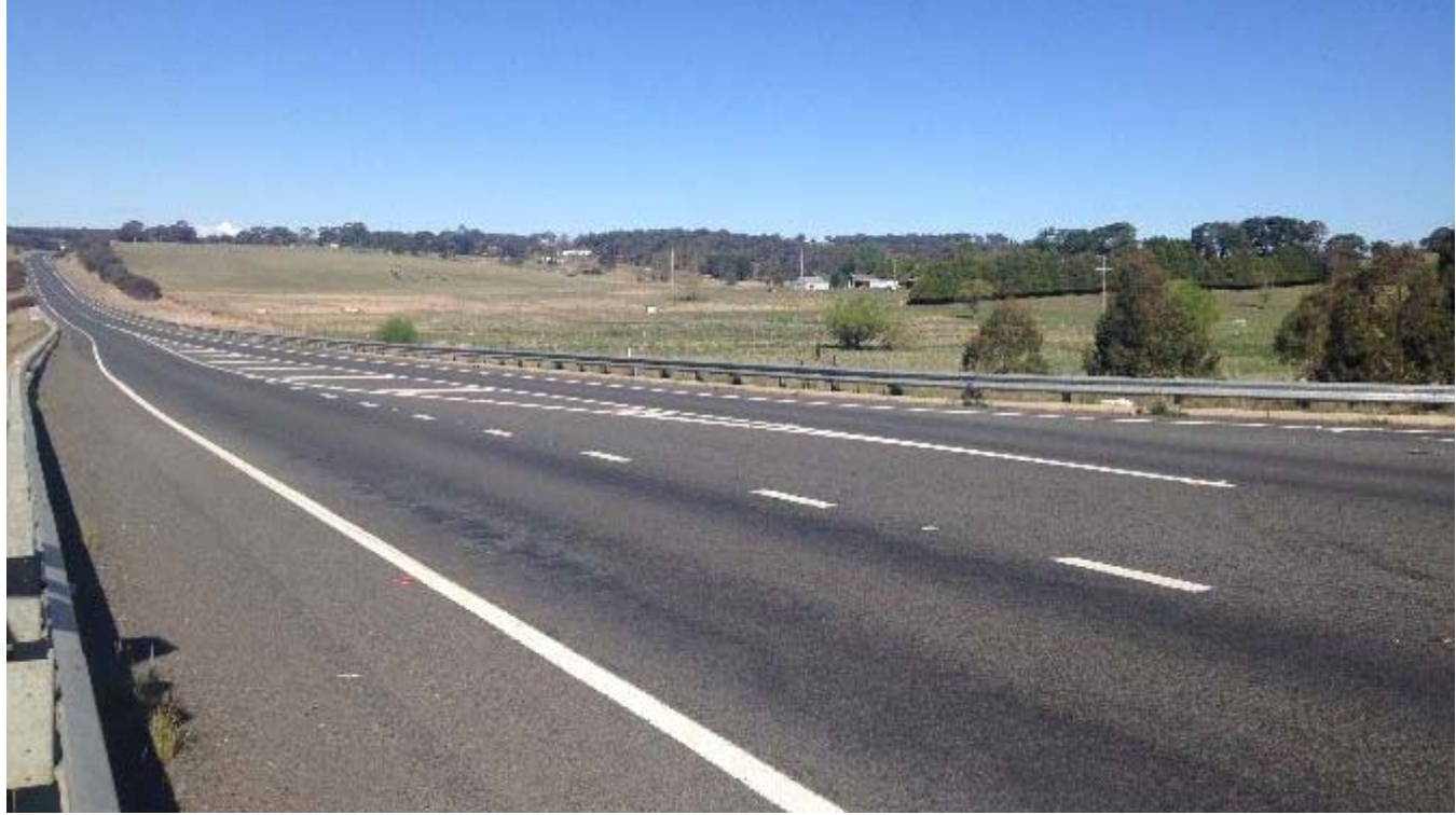
Plate 24: Block cracking, some stripping of aggregate, loss of texture and some deformation
