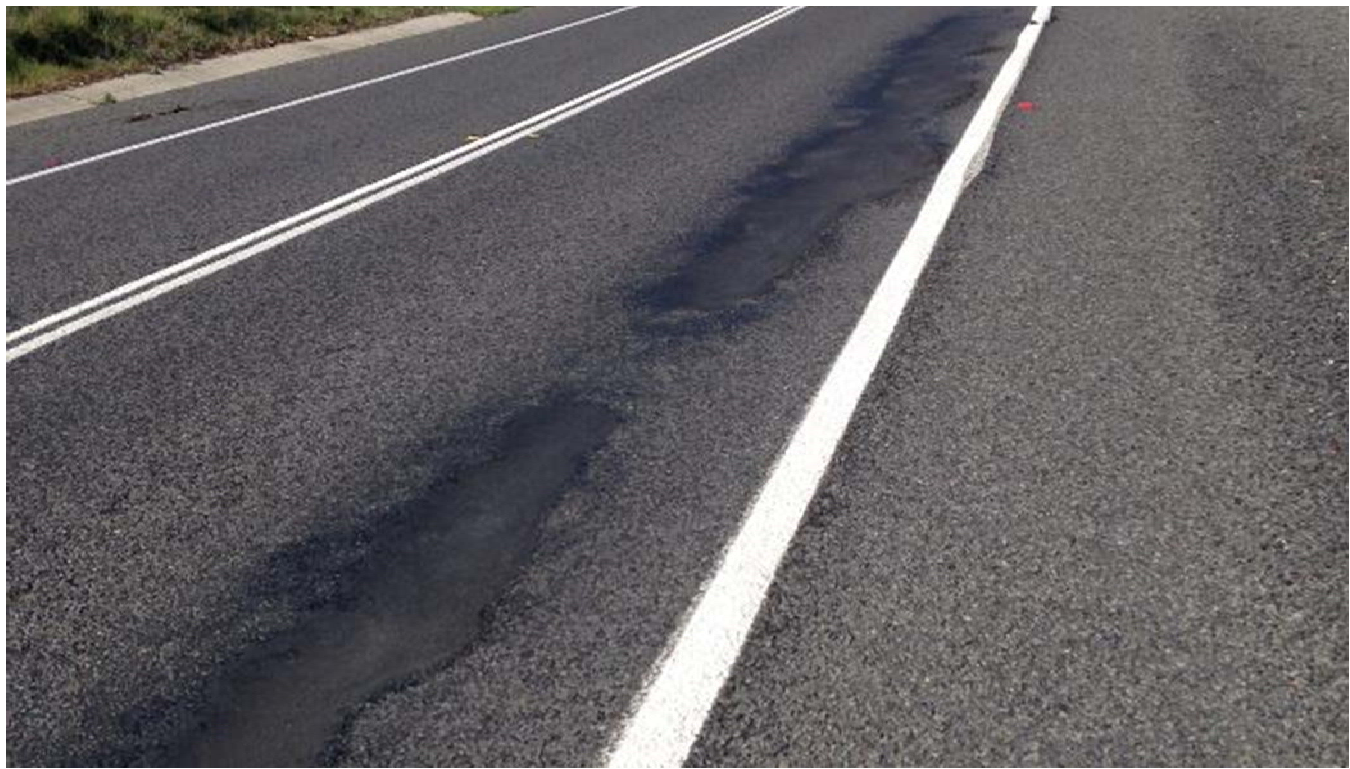
Plate 20: Stripping of aggregate, loss of texture and significant deformation
